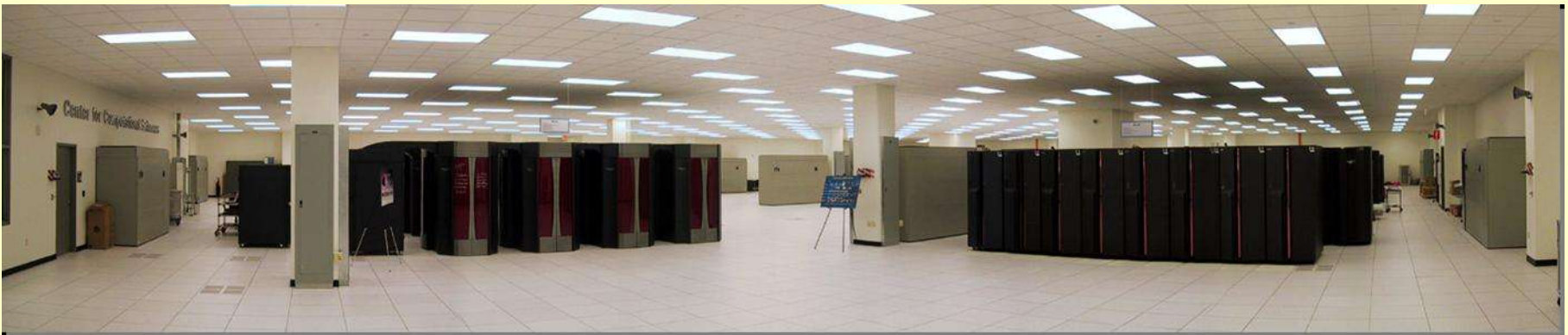
NCCS Facility at ORNL
